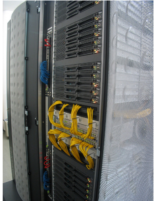
Fig. 14. Tectonic High Performance Simulator (Tethys) with 150 Processors, 150 Gbytes main memory and sustained performance for Earth System models in excess of 300 Gflops. This topical computing system is available to TOPO-EUROPE (courtesy H.P. Bunge).
